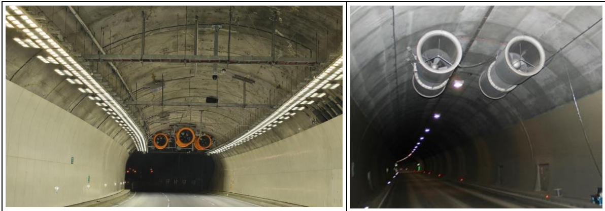
Figure 1: Typical tunnel fitout in Australia (left, Heysen tunnel) and in Austria (right, Niklasdorftunnel [10])
