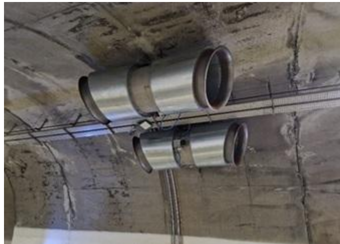
Figure 3: Bank of Jet Fans with Shaped Silencers
