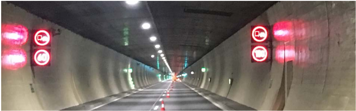
Fig. 1: Example of a faulty display WVZ
