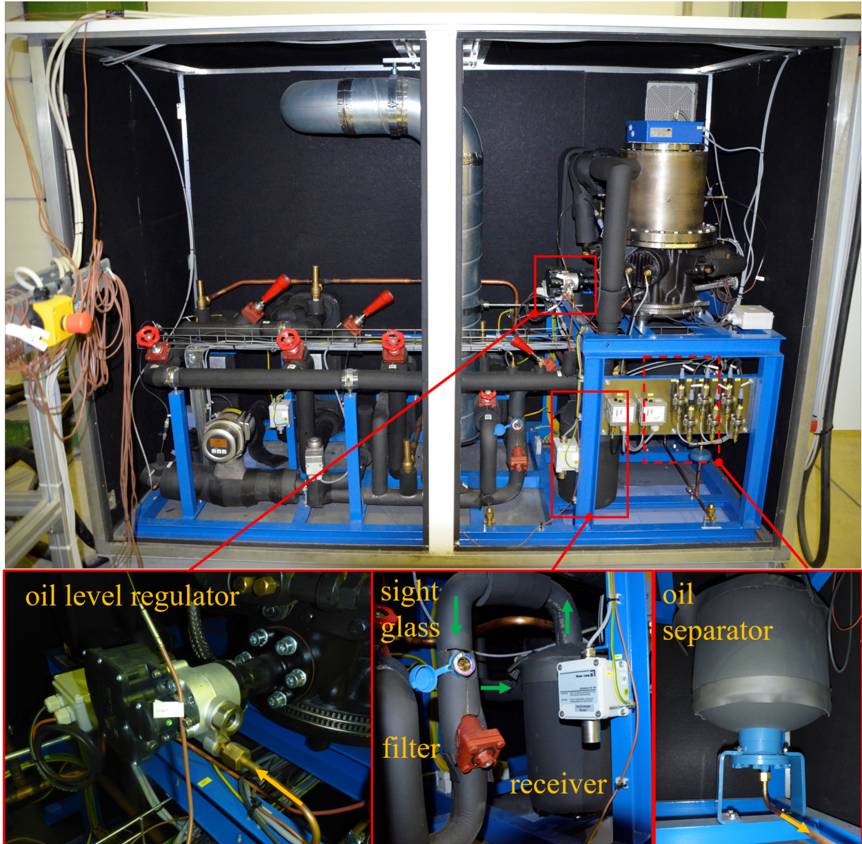
Figure 4.13: Test rig built in situation and component details of oil level regulator, liquid receiver and oil separator
