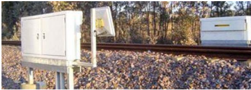
Figure 3-27 - Acoustic automatic inspection system installed alongside a track. Source: [78].
