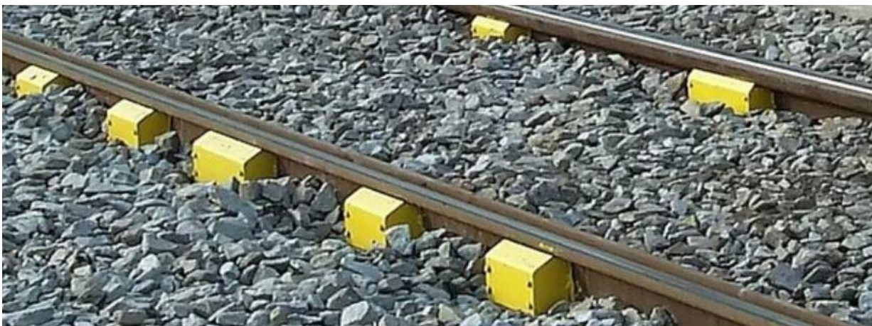
Figure 3-21 - Vibroacoustic sensors installed along the track. Source: [71].
