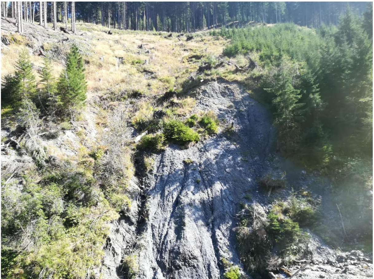
Figure 6-23: Shallow landslide at the eastern slope of the Lorenzerbach at appr. 1200 m. The landslide developed out of colluvium. The proceeding of the landslide can be assumed due to visible scarps in the vegetation at the left side of the picture.
