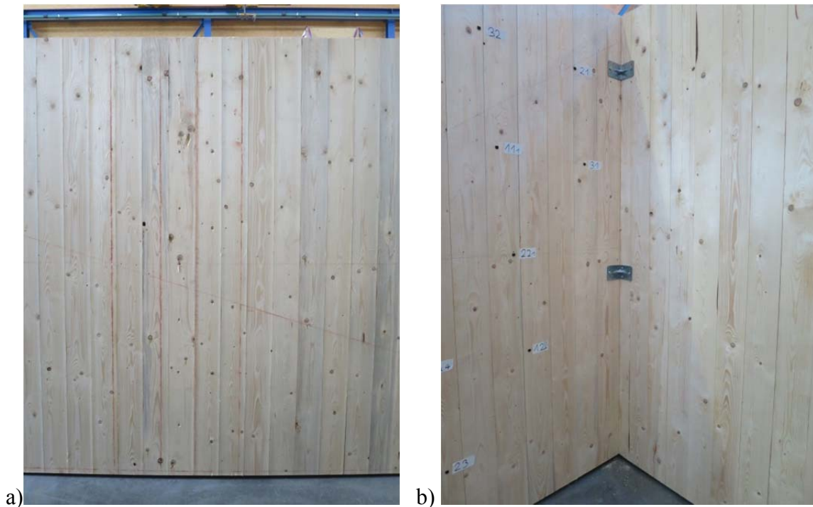
Figure 3.13: Different fastener systems of the used junctions – a) connection using 6 screws; b) connection using 2 angel brackets
