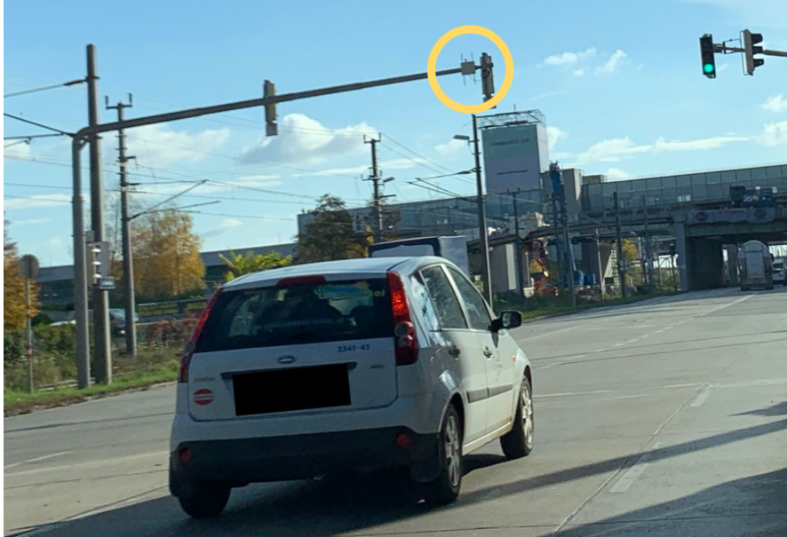
Figure 5.7: Photo of an RSU mounted next to a traffic light at Handelskai and Chrastekgasse
