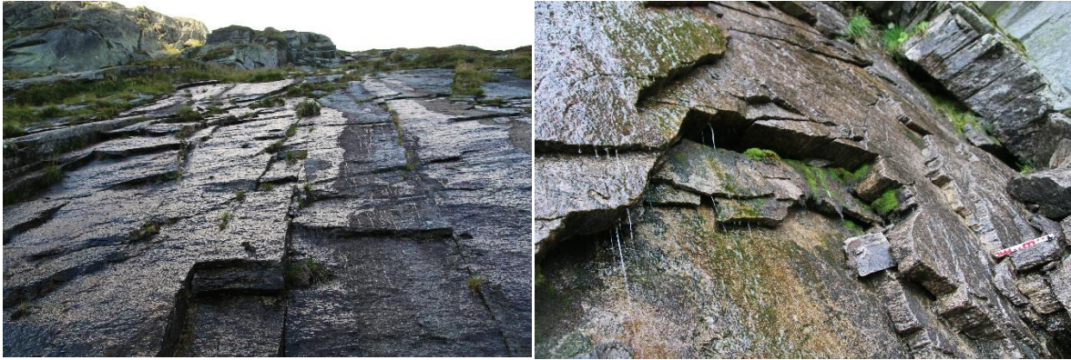
Figure 60 Water flow through very persistent joints. Left through JS1 (Outcrop 4) and right through JS2 (Outcrop 5).
