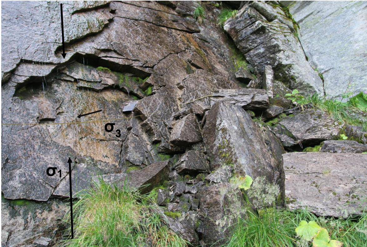
Figure 66 Buckling of rock slabs bounded by sheeting joints.
