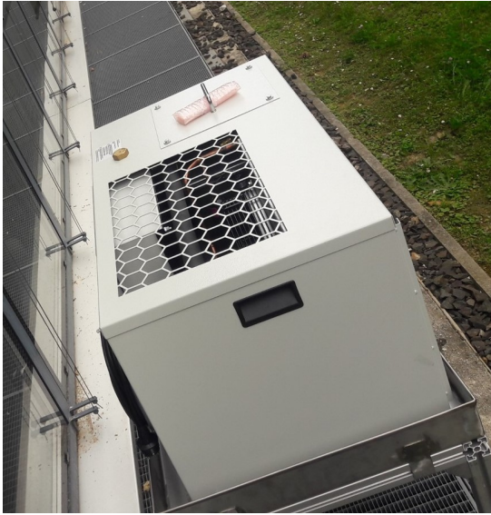
Figure 9: Photo of the external water chiller.
