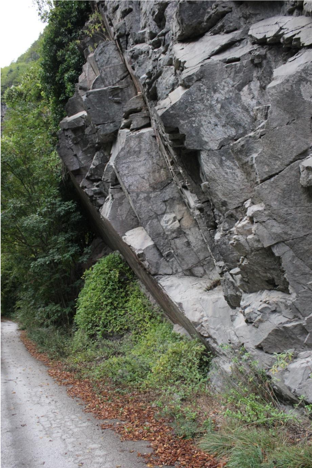
Figure 5: Overview of the typical discontinuities found described in all 4 outcrops for the Gargazzone Fm. That are at least two sets of very steep (sometimes vertical), very persistent discontinuities with one on top and additionally fractures. This creates rectangular blocks, often taking the form of big slabs.
