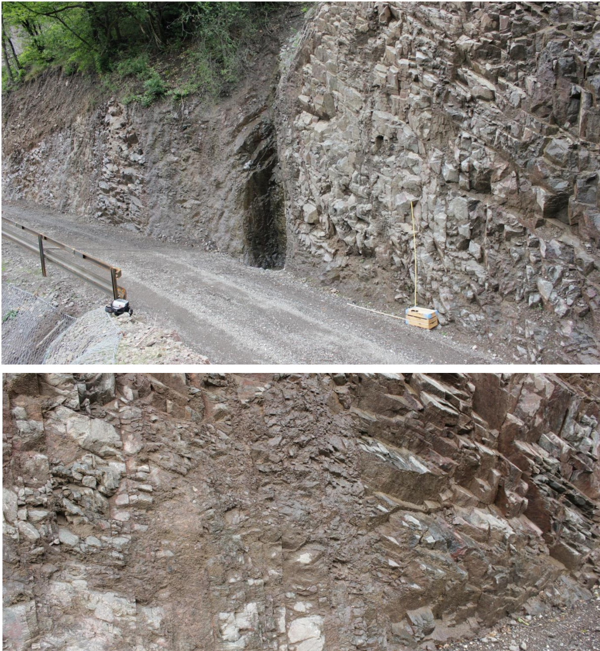
Figure 38: Top; overview picture of the outcrop, most noticeable is the drainage duct in the middle. Bottom; Detail of a highly fractured zone at the upper edge of the outcrop
