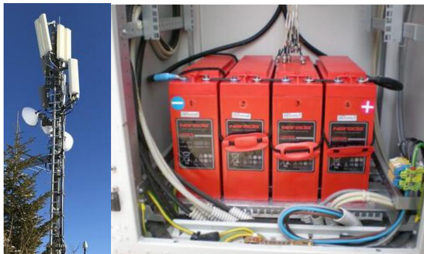
Figure 21: Back-up batteries in Radio Base Stations for mobile services [62]
