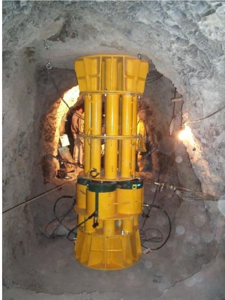
Figure 2.2: Photo of a double plate load test at Khersan II dam site (Rezaei, et al., 2016)
