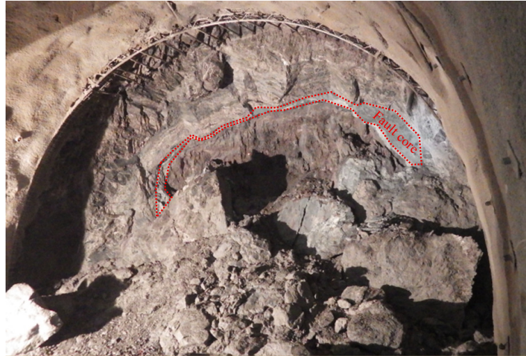
Figure 3.2: Face collapse caused by seepage forces at the Heuberg fault (chainage 921), Semmering base tunnel (ÖBB Infrastruktur AG, 2019)
