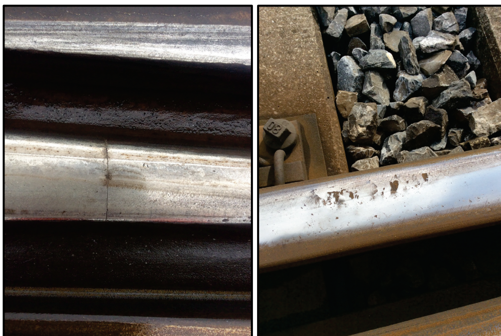
Figure 6.20: Documented defects at T25 reported in ZMON.
