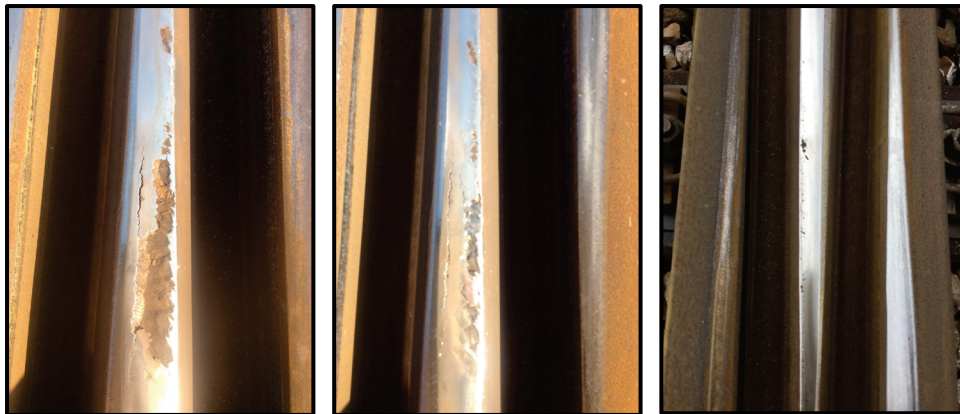
Figure 6.24: Documented defects at T3 reported in ZMON .
