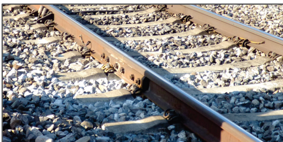
Figure 6.12: Insulated rail joint with characteristic wear pattern after ballast break-up.
