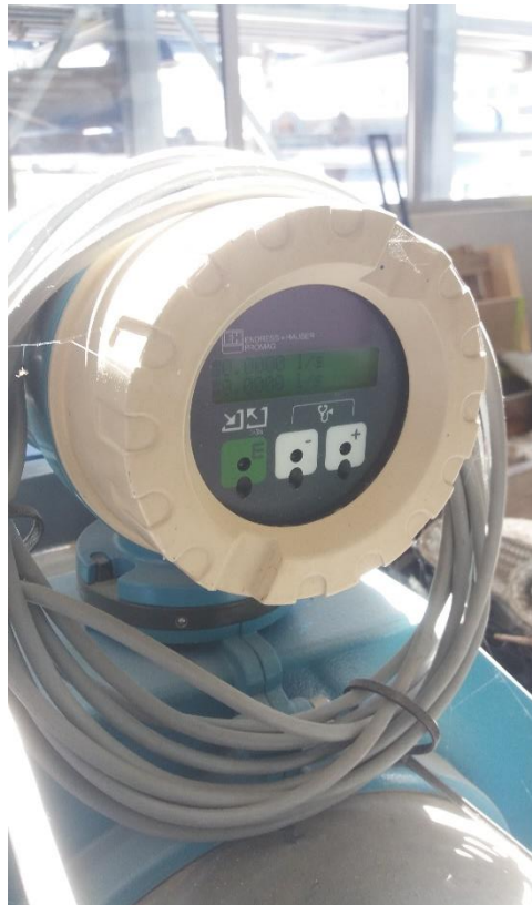
Figure 4.1: Digital meter (MID), to display water discharge Q_w
