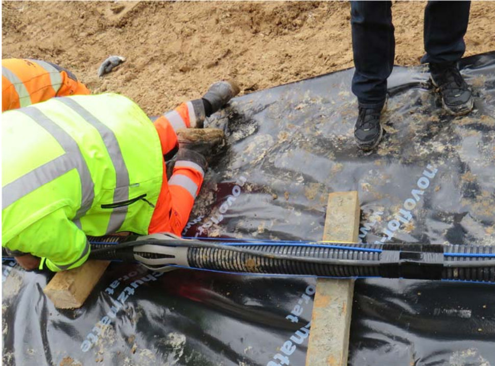
Fig. 104: Fibre optic sensors for grout measurements
