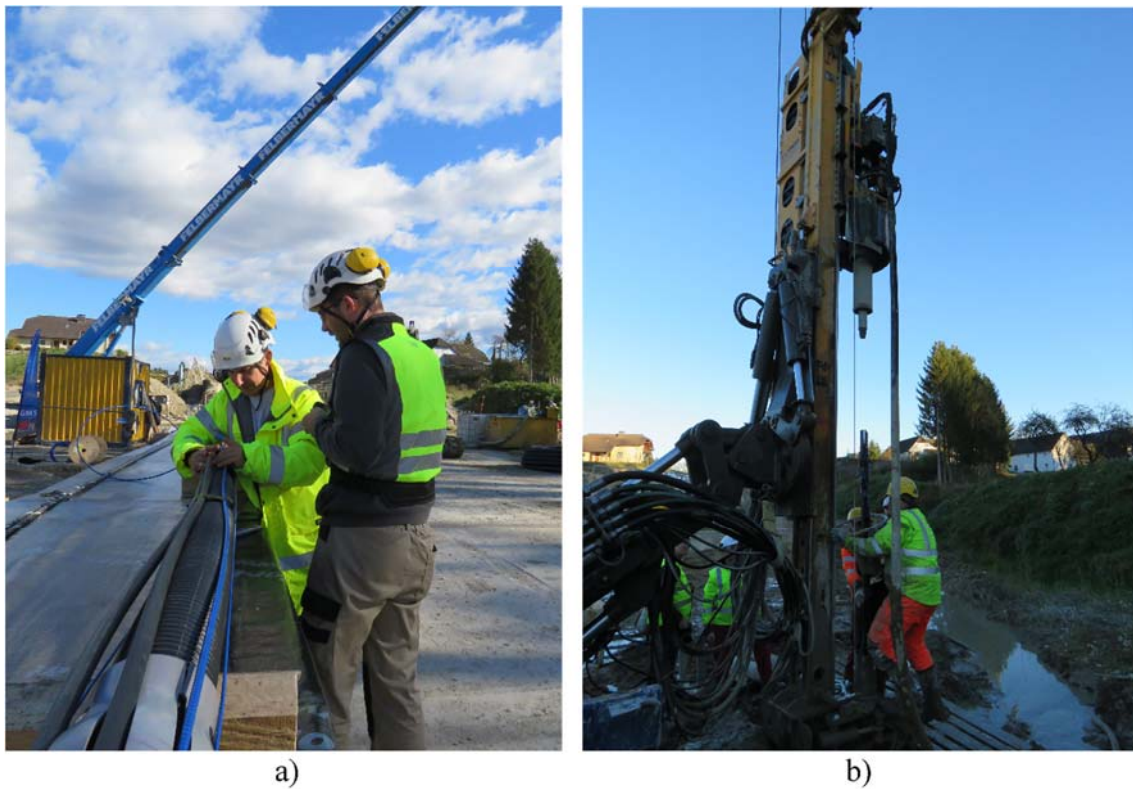
Fig. 30: Anchor 1A – a) fibre optic sensors for grout measurements and b) anchor installation
