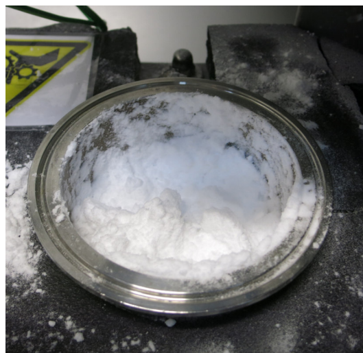
Figure 3.45.: Top view on the material deposit in the connection pipe between rotary valve and lid.
