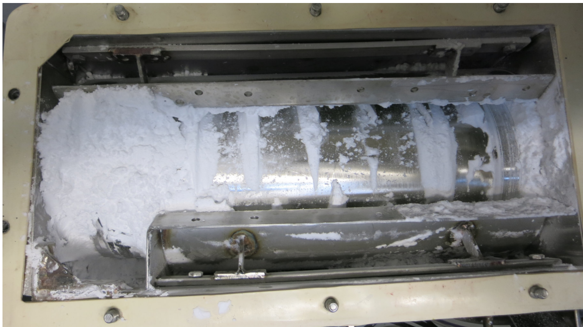
Figure 3.54.: Material inside the dryer at the end of test run V18 without top half shell covers. The material deposit on the inlet was already removed with a vacuum cleaner.
