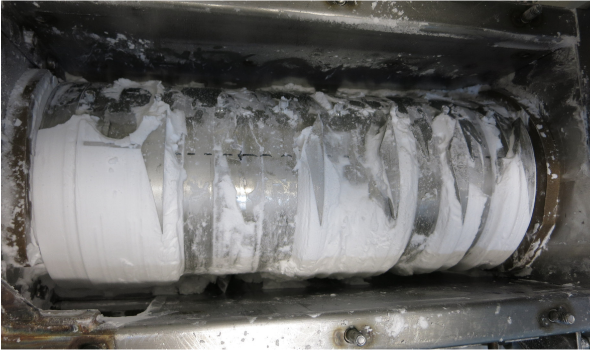
Figure 3.63.: Compacted material deposits on the shaft after removing the half shell covers. Loose material was removed with a vacuum cleaner before the picture was taken. One paddle broke off during cleaning.
