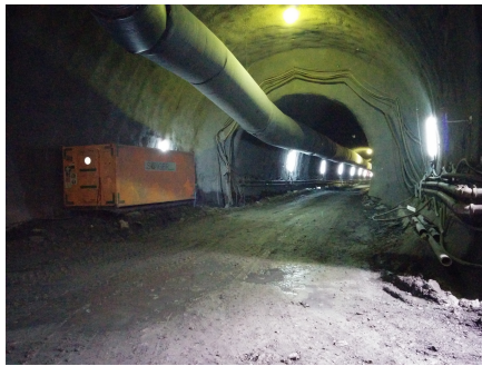
Figure 3.1: Lighting in the exploration tunnel of BBT .
