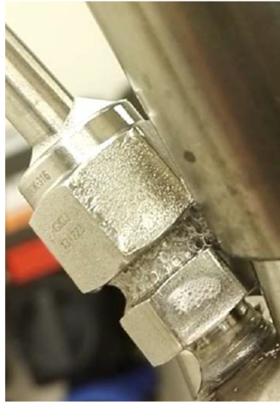
Figure 31: Bubbles of soapy water, caused by leaking gas
