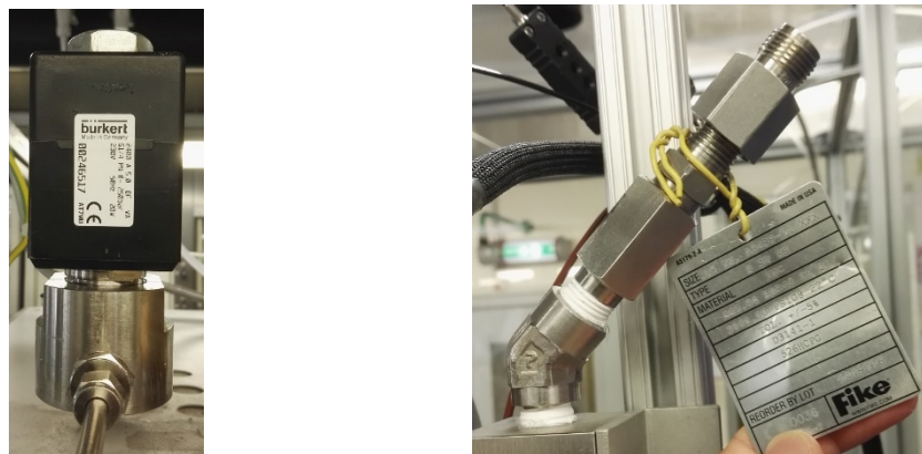
Figure 18: Solenoid valve UV-001, installed in the hydrogen stream and the installed rupture disc SE-001
