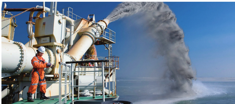
FIGURE 2.3: Placement of fill by rainbowing it from a Trailing Suction Hopper Dredge [6]
