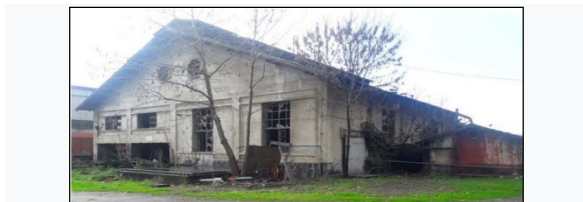
Figure 1: The non-functional Derince Travers Injection Factory
