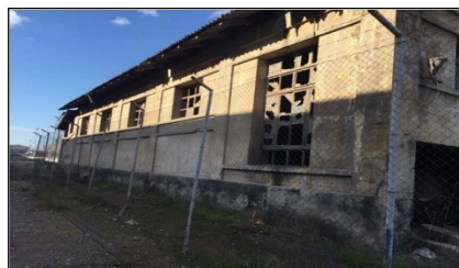
Figure 3: Derince Travers Injection Factory deformation on the facade
