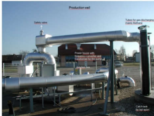
Figure 13, Geothermal system (doublet) in the Austrian town of Altheim, showing its main components, other than district heating piping, source: G. Pernecker, presentation of the project at the Calgary conference [28] 44
