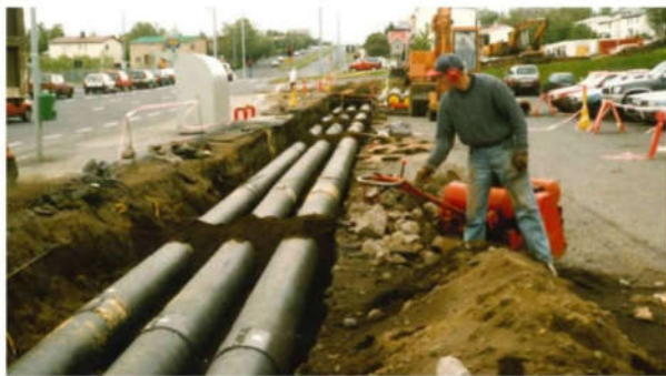
Figure 14, Installment of the Geothermal District heating piping in Iceland, source: www.verkis.is presentation by T. Johannesson, Cornell 2016, used by courtesy of the presenter 45
