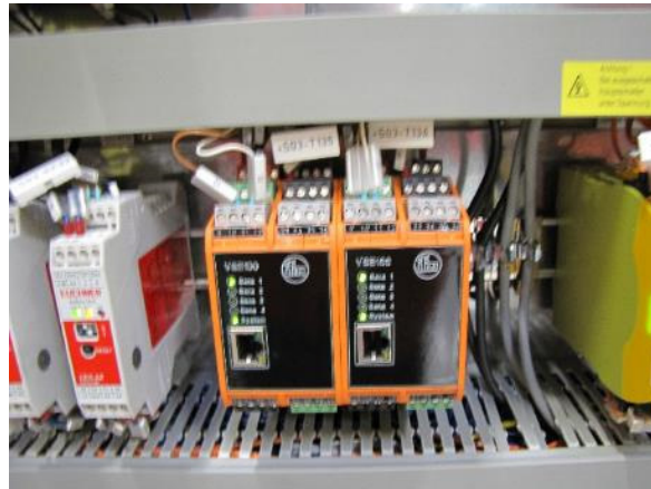
Figure 40: Already installed diagnosis system
