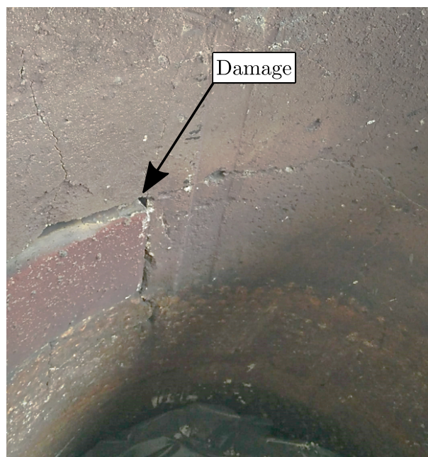
Figure 7.14.: Damage at the inner walls of a regenerative casing seen during annual shutdown.
