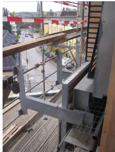
Figure 4: Installed Steel Fin
