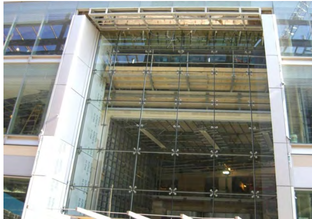
Figure 7: Explosion resistant cable net façade, Court square project, long Iceland, United States (Gartner)
