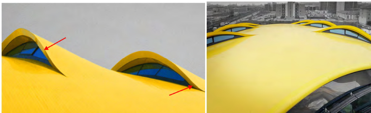
Figure 9: Metal cladding at the skylights. The red arrows indicate zones of strong double curvature. (Teleya)
