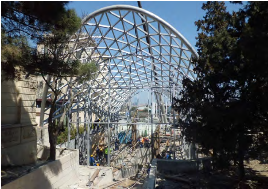
Figure 9: Assembly valley station
