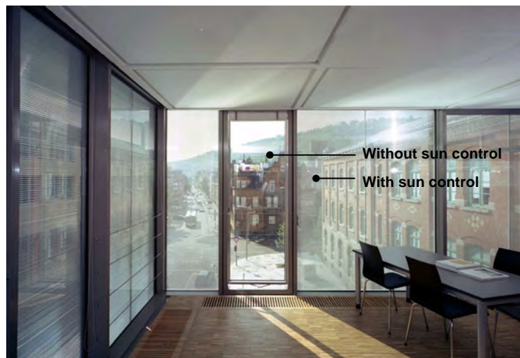
Figure 12: Integral sun control system at the façade of the Landesdenkmalamt Baden-Württemberg, Esslingen.
