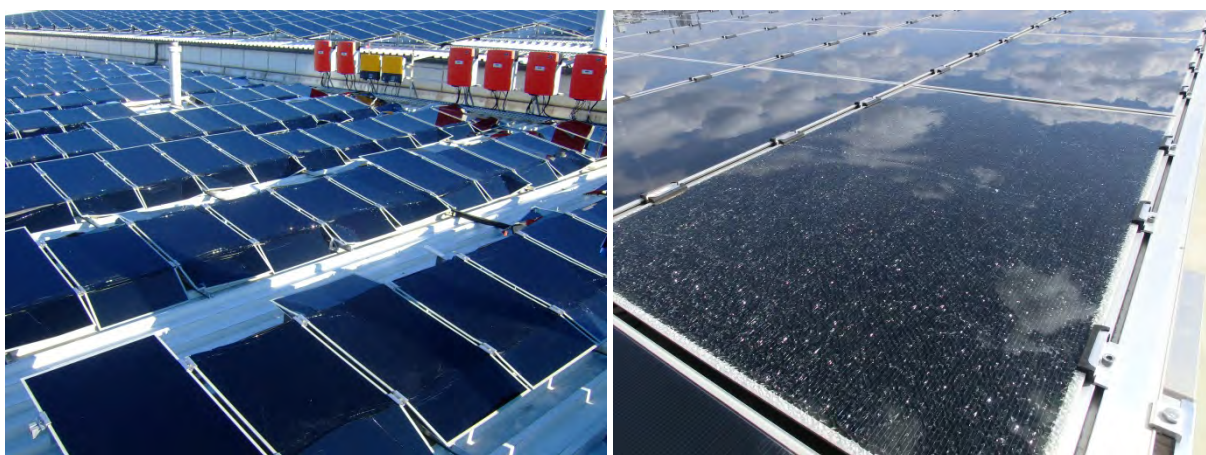
Figure 1: Damage pattern in thin-film PV modules with glass-glass assembly
