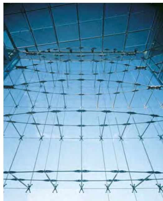
Figure 4: Cable net facade with polygonal cable direction (type 2): Sony Center, Berlin (Gartner)
