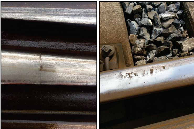
Figure 47 Documented defects at T25 reported in ZMON .
