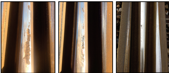
Figure 51 Documented defects at T3 reported in ZMON .
