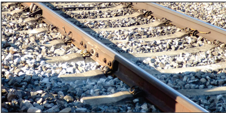
Figure 39 Insulated rail joint with characteristic wear pattern after ballast break-up.
