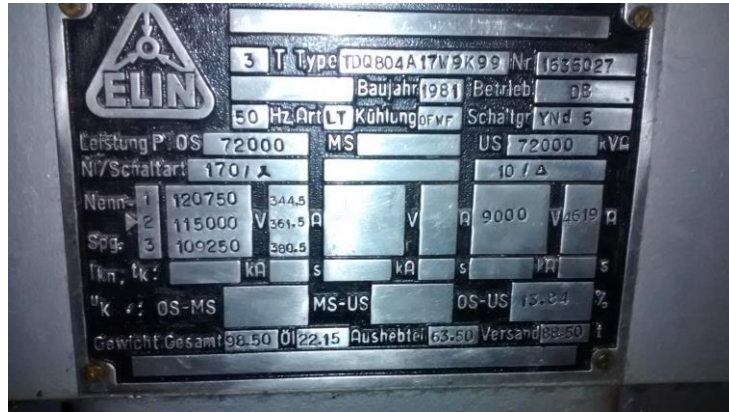
Figure 7-1: Transformer specification plate
