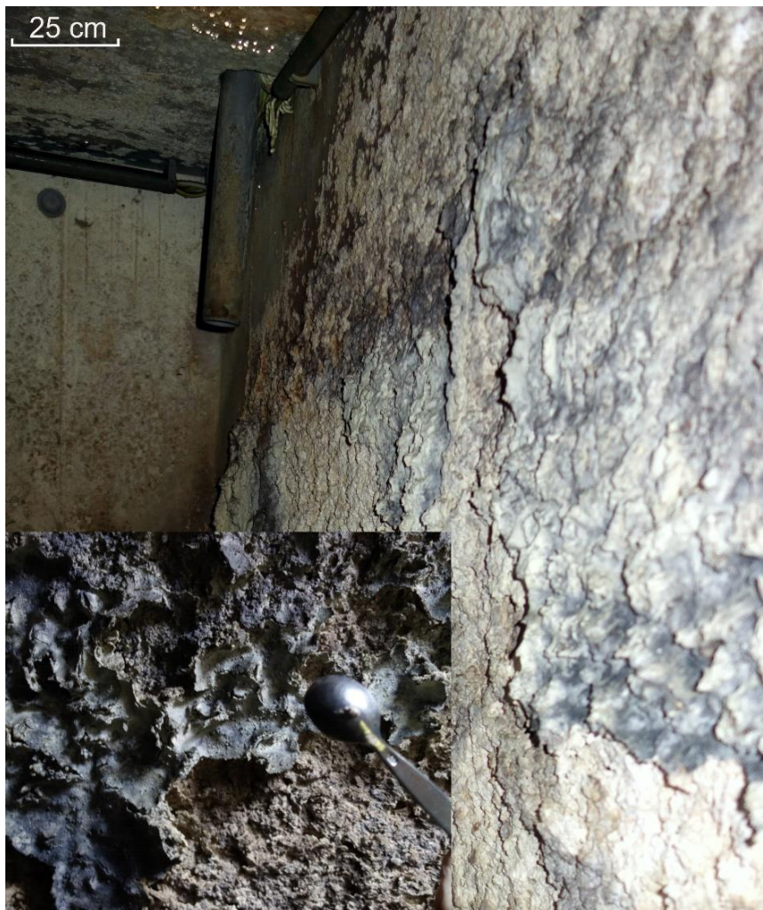
Figure 1: Strongly deteriorated concrete walls of a sewer system affected by MICC. The outer surface consists of a material with no internal strength which can be wiped away easily with a small spoon (detail photo bottom left).
