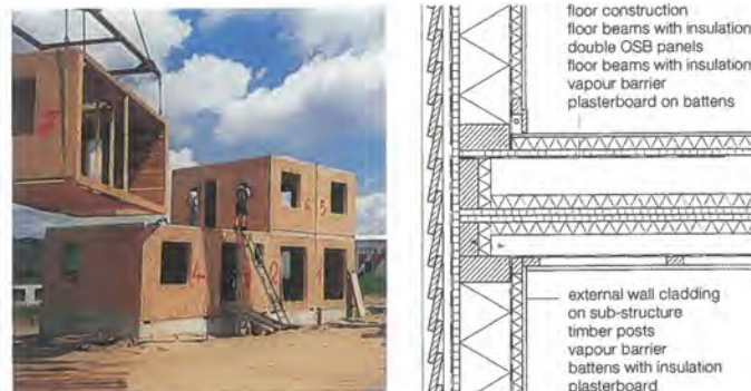
Figure 2-50: Transport and assembly of timber building modules and a section through the module. 101
