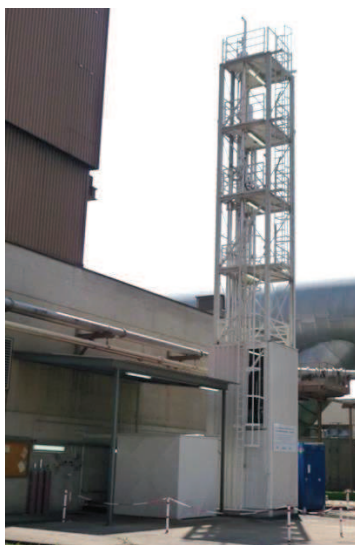
Fig. 5-3. Overview of the CO 2 SEPPL pilot plant.
