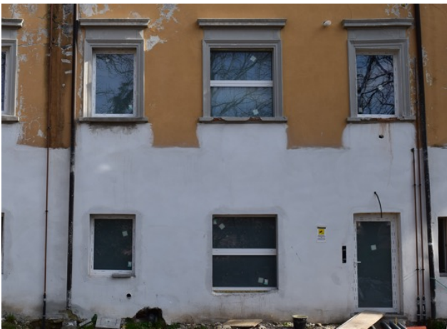
Fig. 6: picture taken in Gorizia to a similar building where no attention is paid in preserving both authenticity and integrity of the façade.
