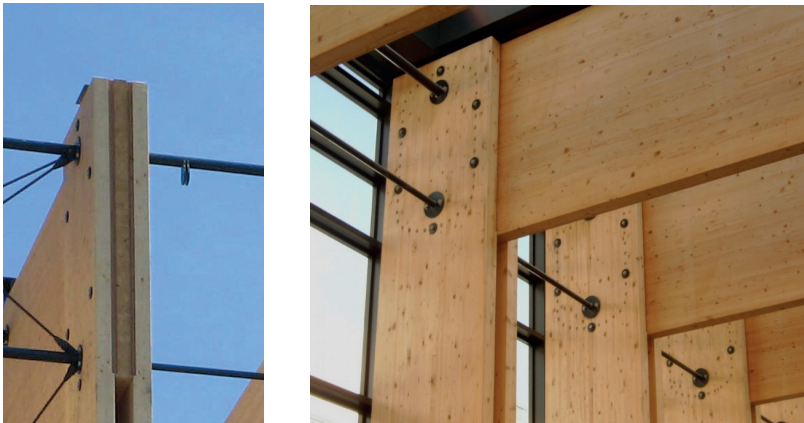
Fig. 7 Reinforced two-hinged frame with dowel circle (UCD Dublin Library, 2005). Plywood board (beech) 4 x20 mm fully glued on both sides (columns and crossbar) to avoid cracks
