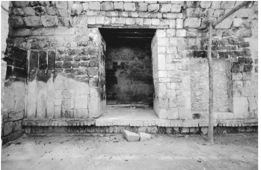
Fig. 138 The reused cornice elements of the upper member of the three-member base molding in Room 9 under the southern wall. Photograph: H. Hohmann 2004
