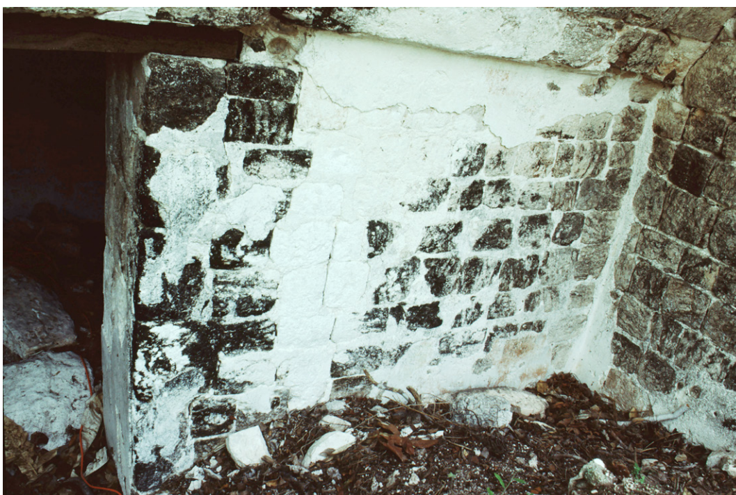
Fig. 163 The wall north of the passageway shows two bands under the vault spring with remains of Maya hieroglyphs and remains of a mural representing at least four persons above the rubble. Colors: brown, green, and orange. Photograph: J. Sulak 1989
