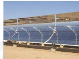
Abengoa Solar - Trough collector
