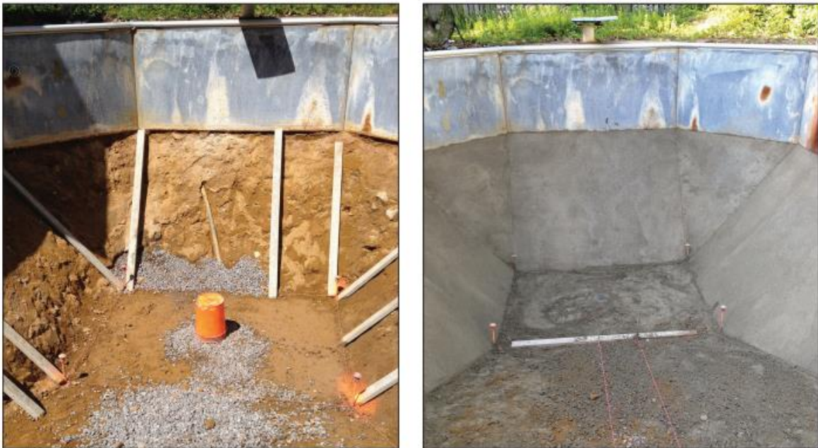
Figure 20. Refurbishment of an outdoor in-ground pool with (insulating) perlite-concrete pool bottom (perlite.org)
