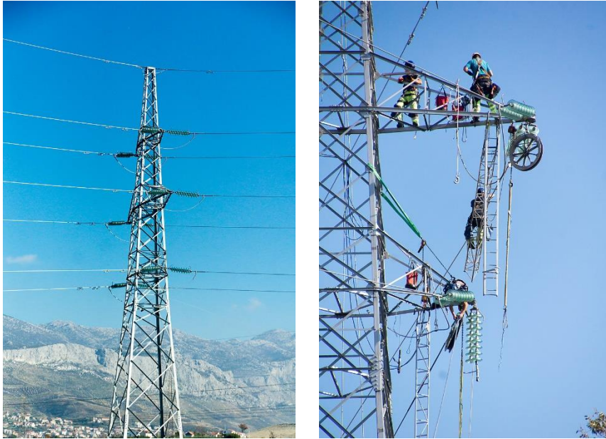
Figure – Reconductoring Project in Split network (HOPS, Croatia)
