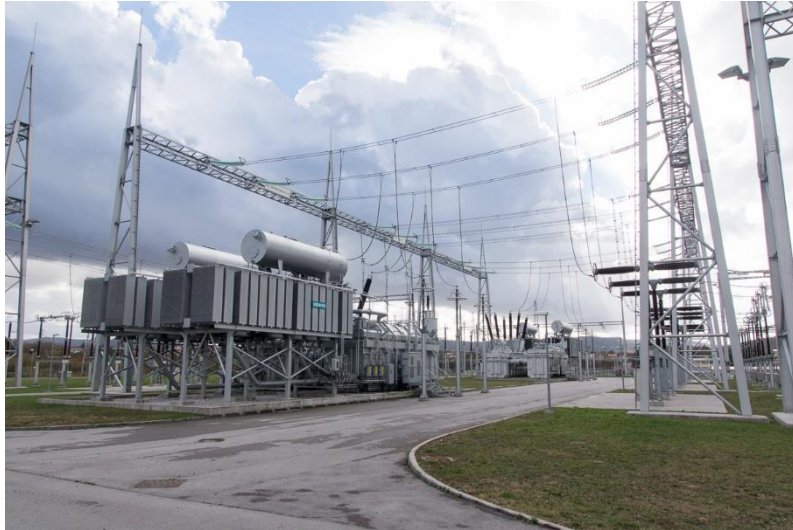
Figure 6.3 – PST 1 (foreground), PST 2 (background) in SS Divača (ELES, Slovenia).
