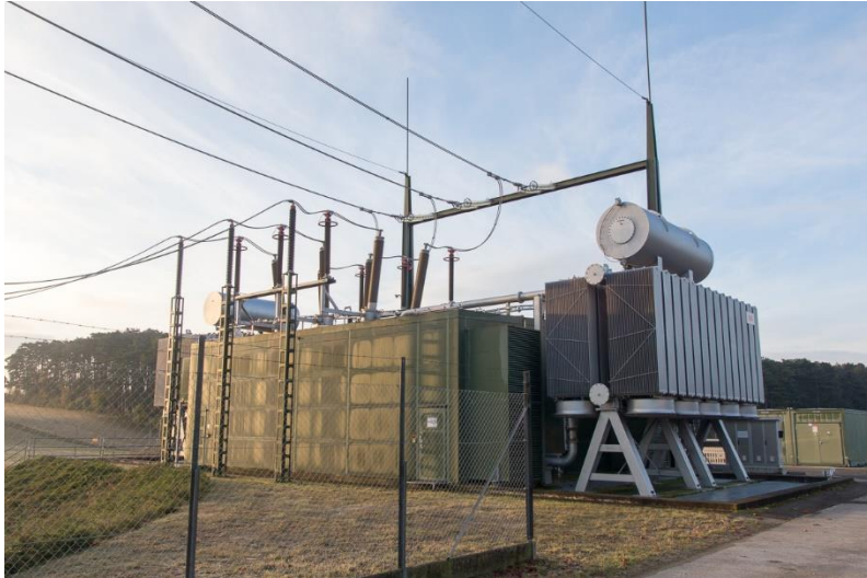
Figure 6.9 – PST in SS Ternitz (APG, Austria)
