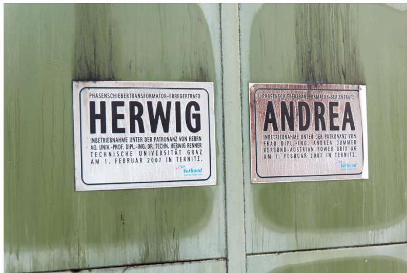
Figure 6.10 – Nameplates of PST in SS Ternitz (APG, Austria)
