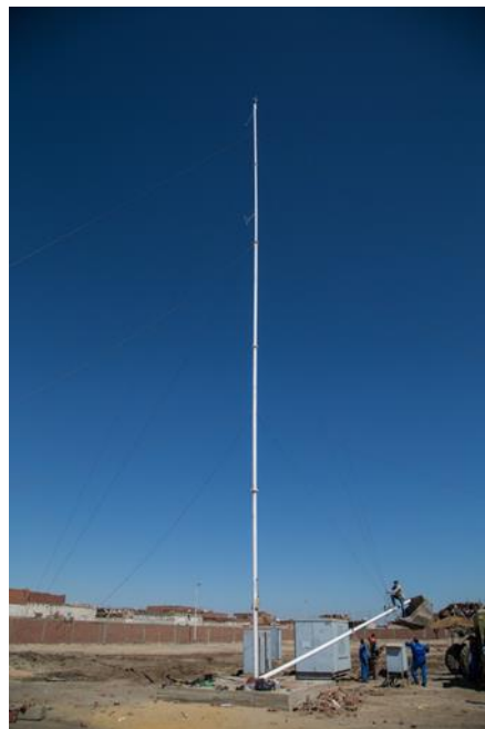
Figure 32: The wires from the gin pole were fixed at the anchor, when the mast was fully upright
