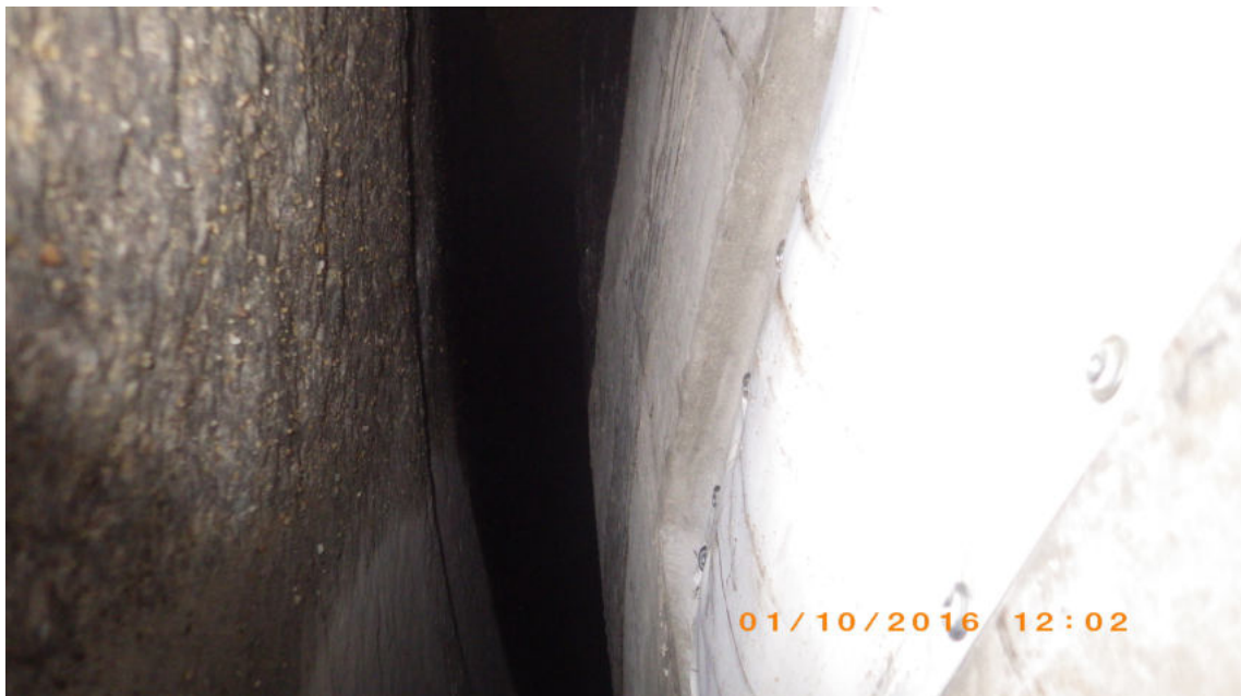
Figure 74: Geotextile tube embedded into the lining segment prior to the injection (taken from Henzinger et al., 2018).
