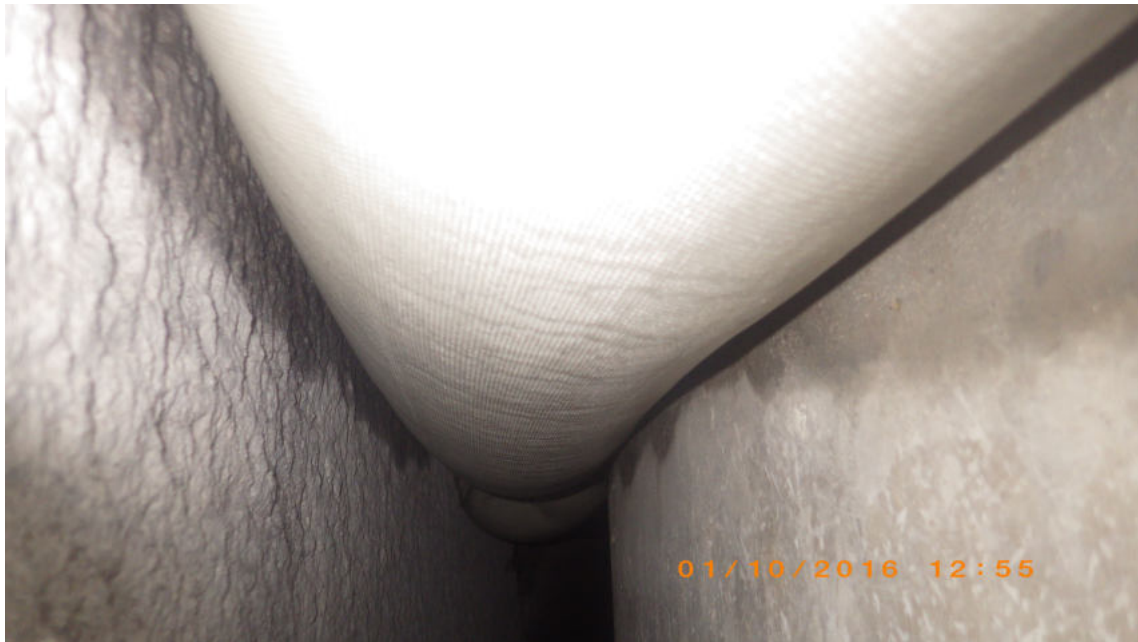
Figure 75: Geotextile tube after the injection with full contact to the excavation boundary (taken from Henzinger et al., 2018).
