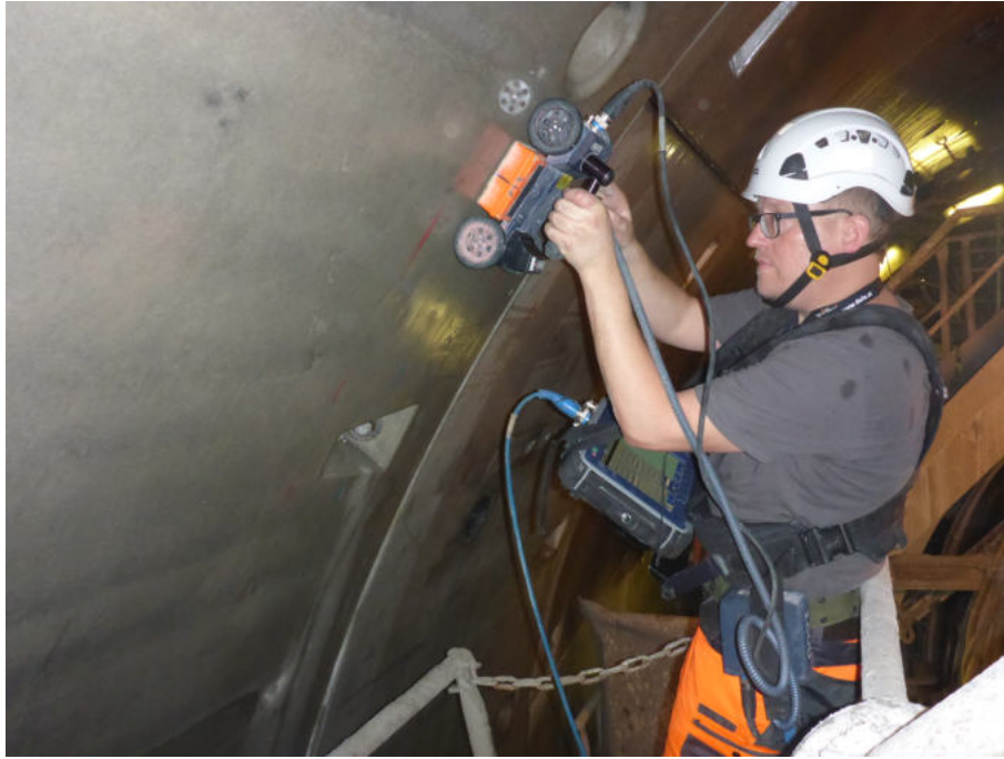
Figure 58: GPR measurements for the void detection in the annular gap at the south tube of the Koralm tunnel construction lot KAT2.
