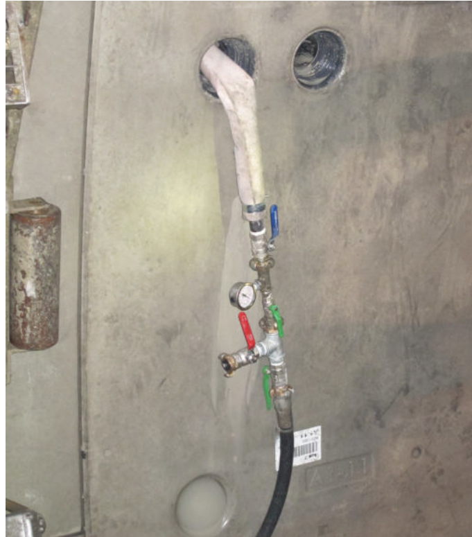
Figure 72: Additional opening for the injection of the geotextile tubes next to the pea gravel openings (taken from Henzinger et al., 2018).
