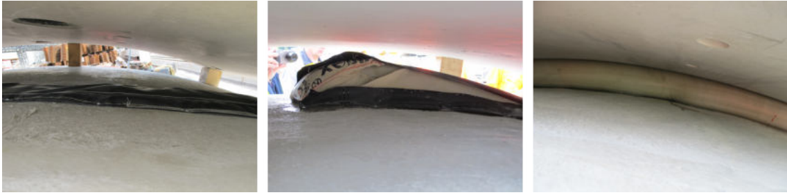
Figure 70: Filling process of a Bullflex ® geotextile tube between two lining segments; left: state before inflation, middle: geotextile tube during the inflation process, right: fully inflated geotextile tube (taken from Henzinger et al., 2016).
