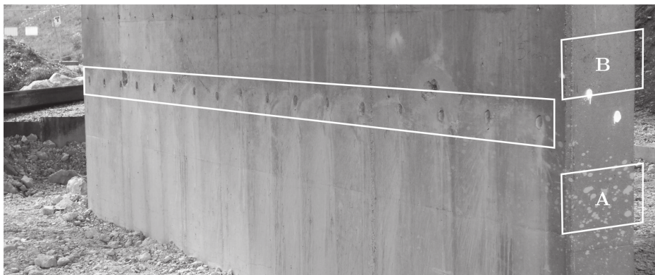
(c) introduced damage of pillar between monitoring areas A and B
