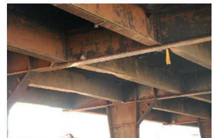
[Figure 128] Deformations on Fevkani bridge.
