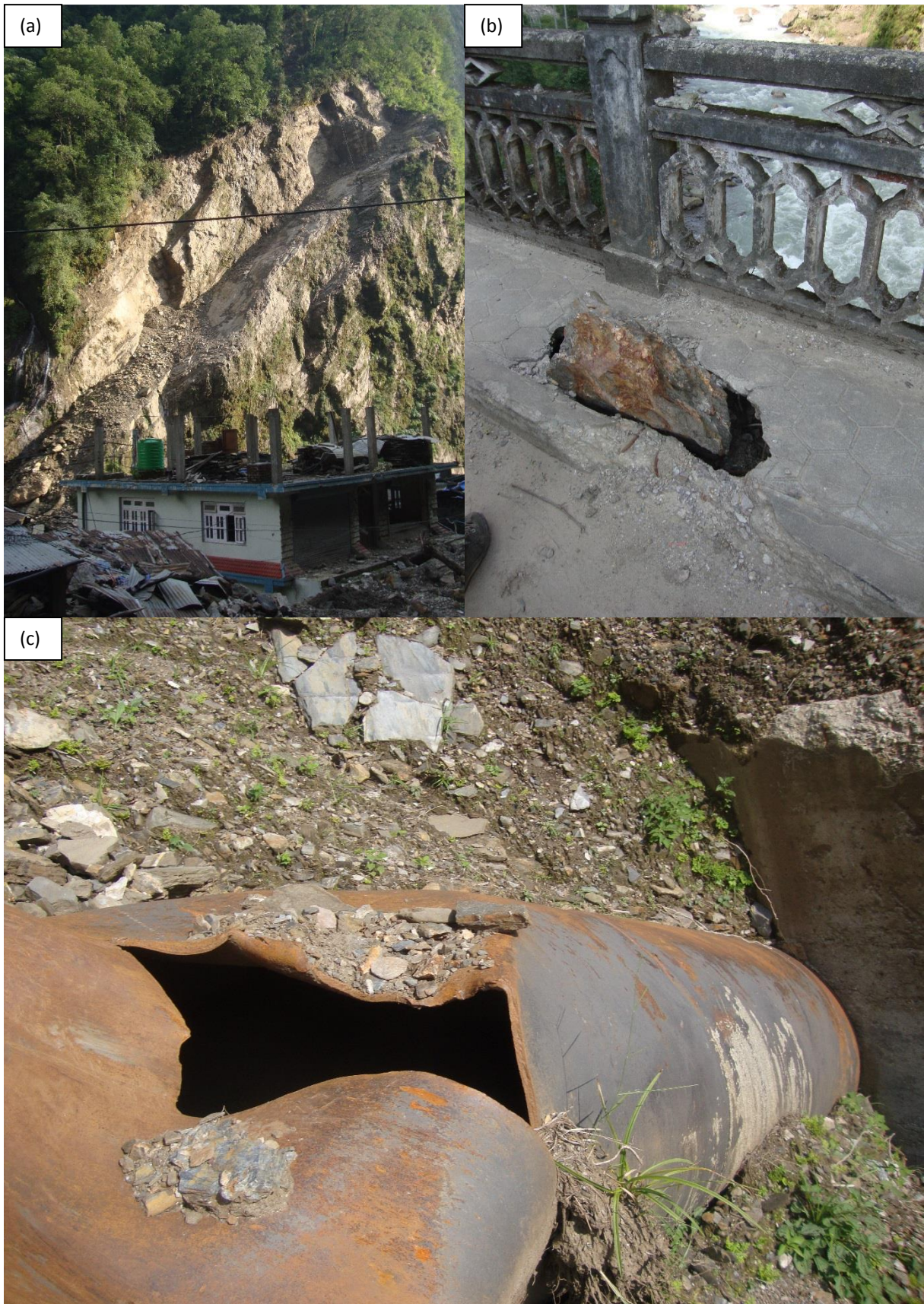
Fig. 63: Images showing the influence of earthquake induced landslides on infrastructure; (a) Influence on houses (foreground), rock slide on fault surface (background) (27.93446° N, 85.93931° E); (b) Influence of rockfall onto bridge / road (27.93077° N, 85.93637° E); (c) Influence on waterpower plant pipe (27.93386° N, 85.93732° E)
