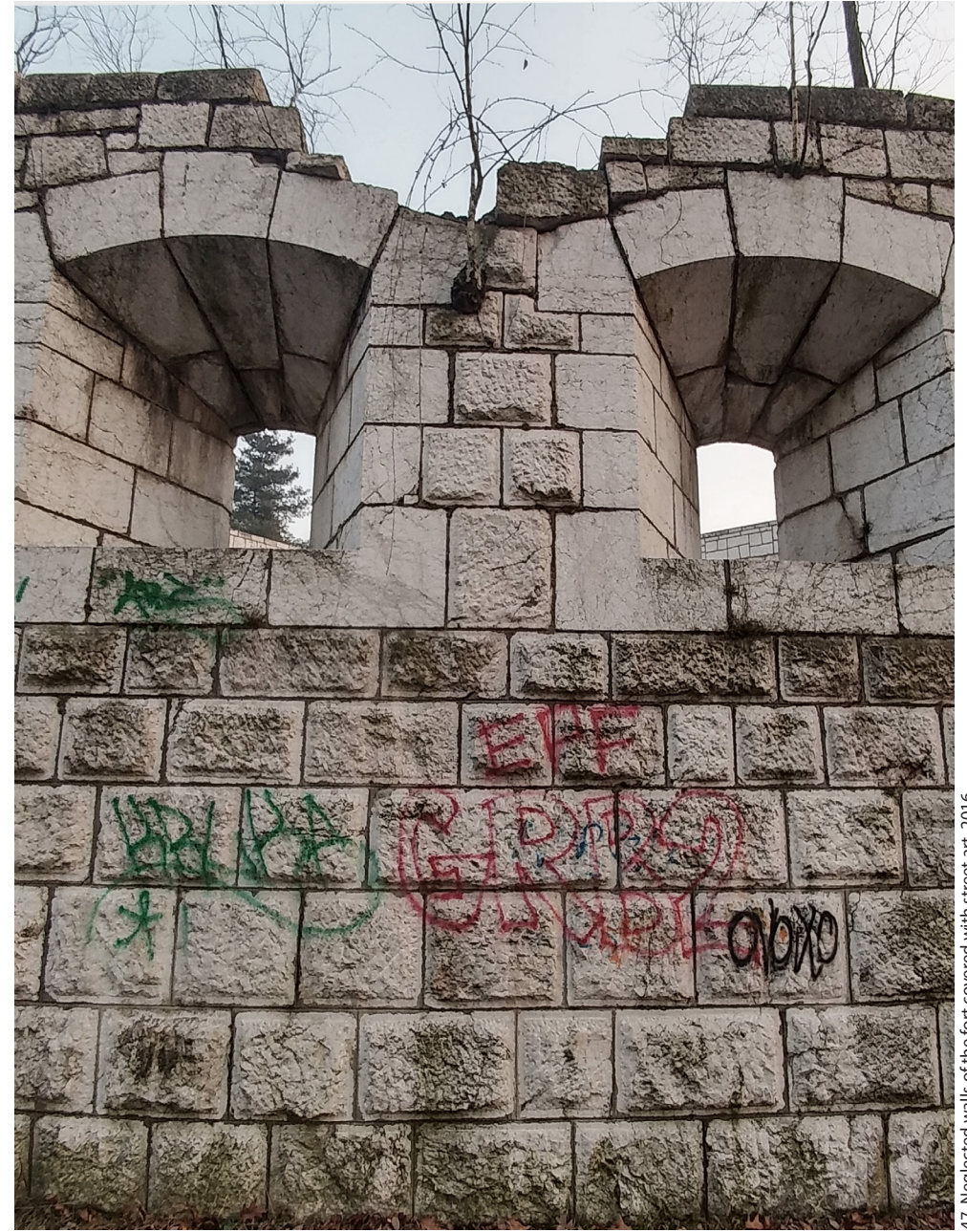
47. Neglected walls of the fort covered with street art, 2016
