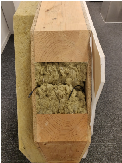
(a) Sensors are placed within the wall of an exterior wall.
