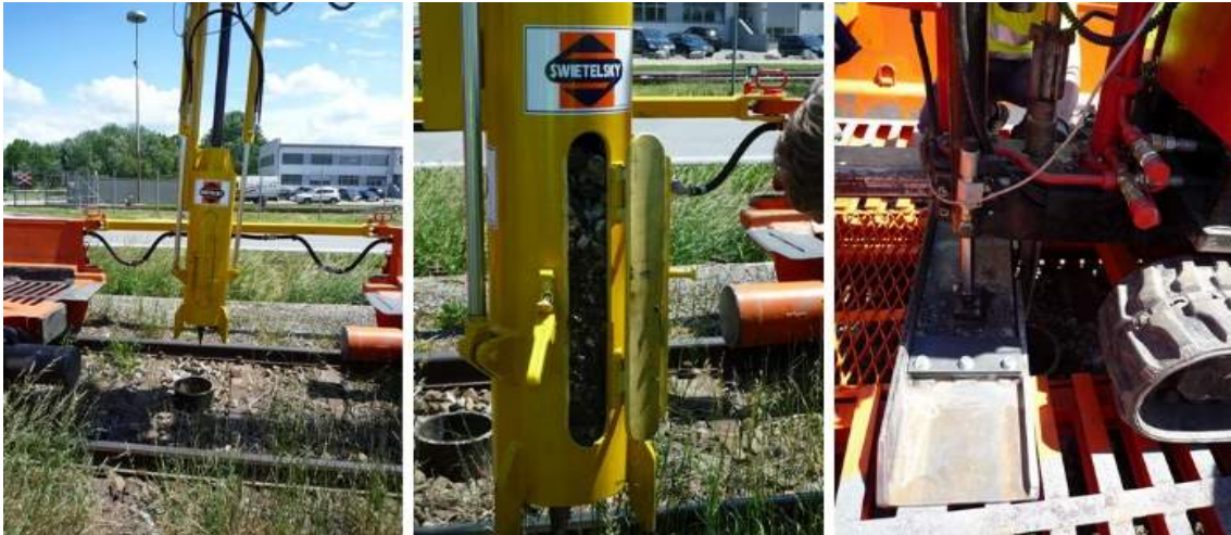
Figure 29 Track-bound CPT (left: cladding tube driven in by vibration, centre: ballast extraction, right: pressure sensor)
