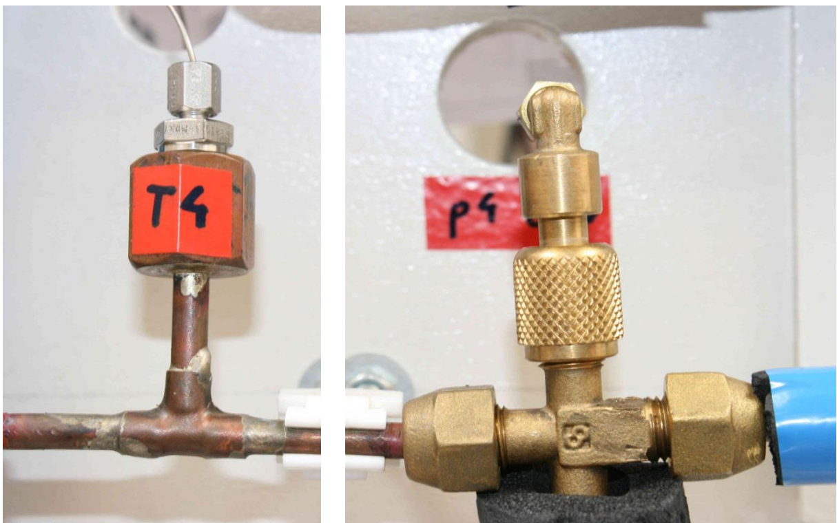
Fig. 52 Measuring points of pressure (right) and temperature (left) before being insulated.
