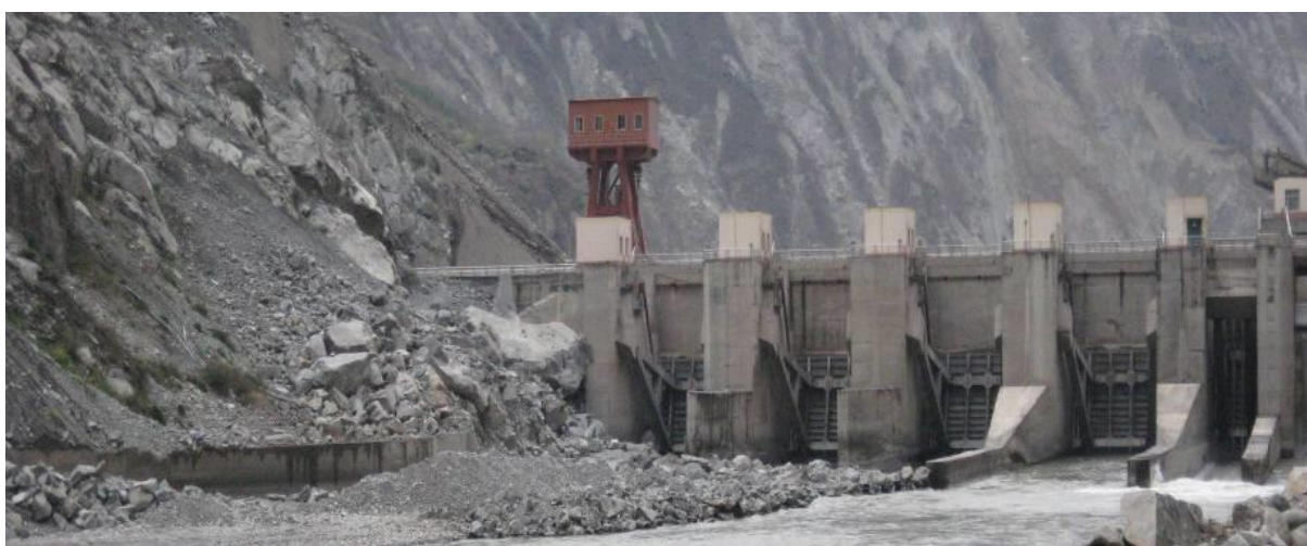
Figure 3: Damage of spillway piers caused by rockslides during the 2008 Wenchuan earthquake in China
