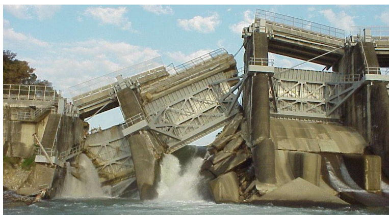
Figure 2: Failure of two bays of the Shih-Kang weir caused by (mainly vertical) fault movements during the 1999 Chi-Chi earthquake in Taiwan
