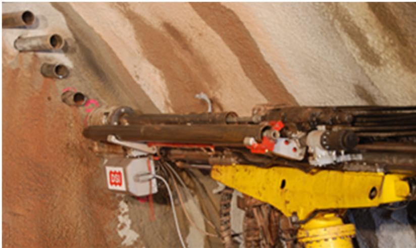
FIG 3. Piecewise installation of a pipe umbrella drill under limited space conditions in a conventional top heading-benching excavation.
