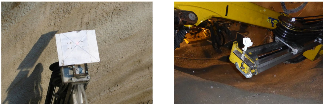
Figure 10. Different types of targets at the end of a drill arm. Both work but the left one has advantages because the bigger area eases to find the laser light
