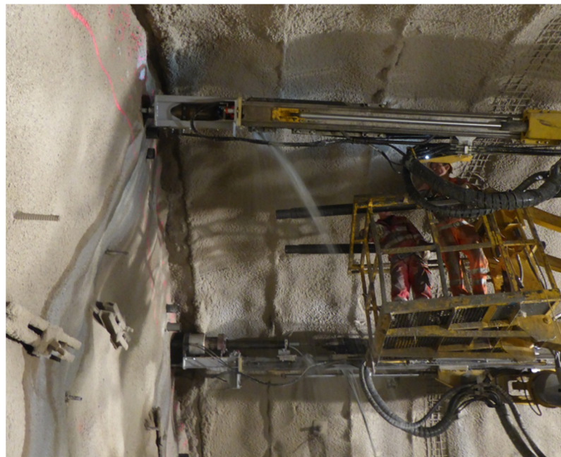
FIG 9. Pipe umbrella installation with two squeezing units mounted onto the drill booms during drilling and a feeding lifter in the middle.
