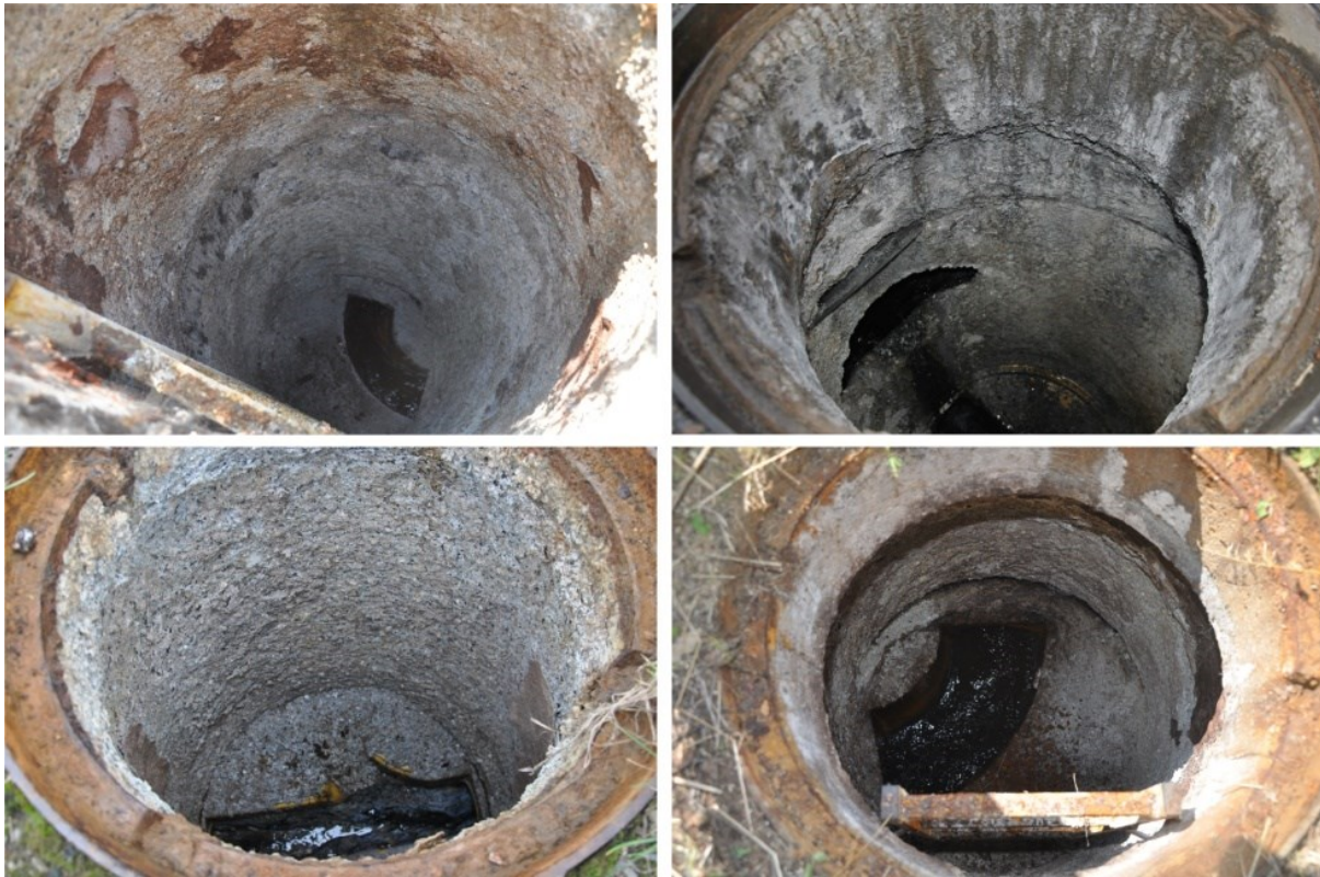
Figure 1: Typical damage pattern of MICC from different Austrian sewer manholes.
