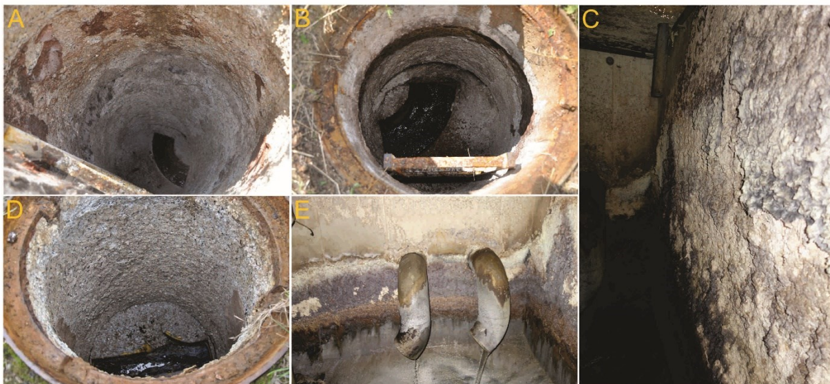
Figure 1: Examples of typical deterioration symptoms within systems affected by microbial induced concrete corrosion. Pictures A, B and D were taken in concrete manholes following a power main, while pictures C and E display damages within wastewater catchment basins. For details regarding system and concrete.
