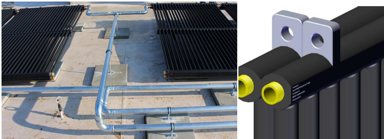
Figure 3-3: Picture and scheme of the installed solar collector; left (Projekt HOT ICE, 2017) right (Viessmann, 2017)
